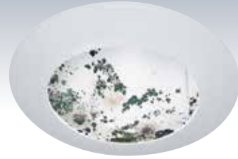
Ingress of Mold
